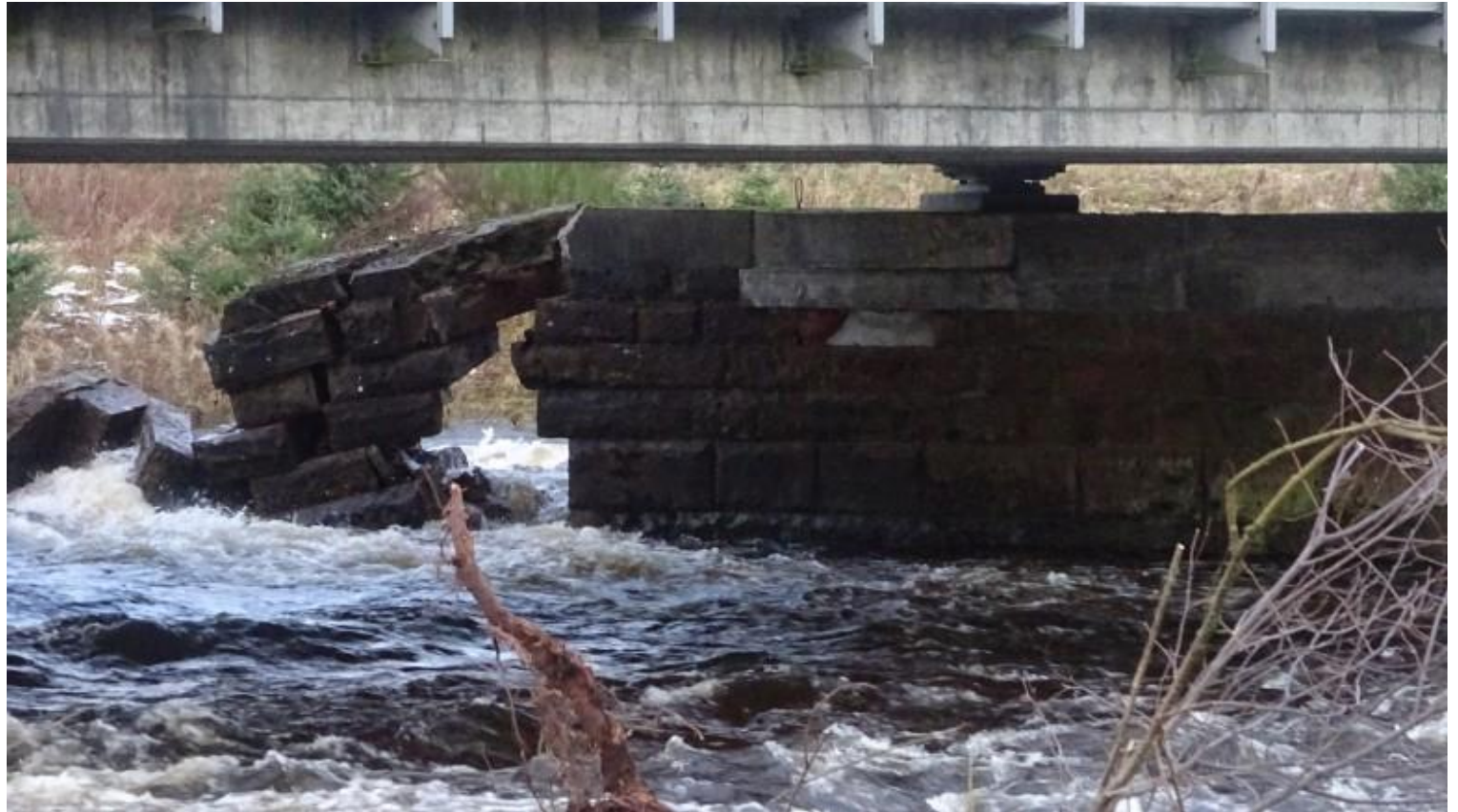
Effects of Bridge Scour, Lamington Viaduct – 31 Dec 2015
